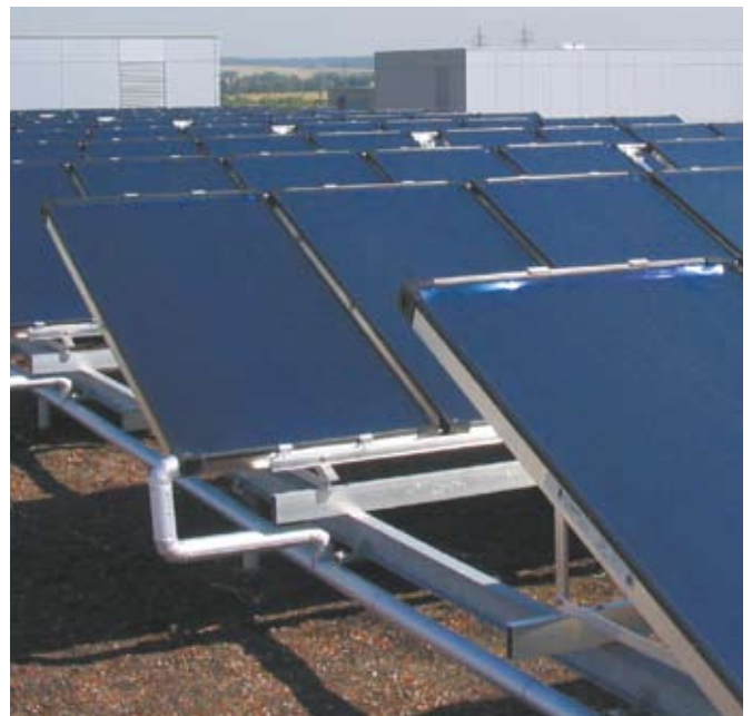
Typical BT collector field
